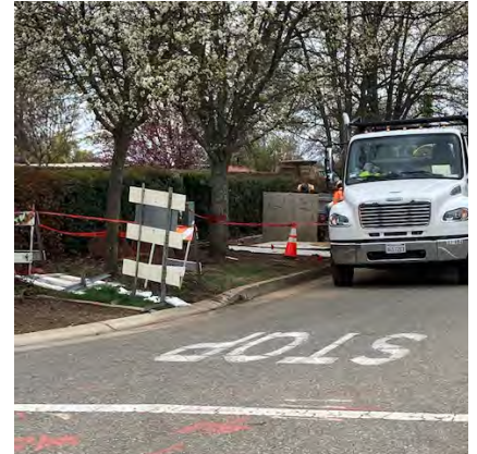
Bass Lake Road at Madera Way Construction (photo credit - Tasha Boutselis Camacho)
