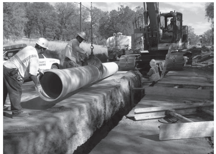
New 20-inch diameter PVC pipe goes into the ground to replace a portion of the Motherlode Force Main.
