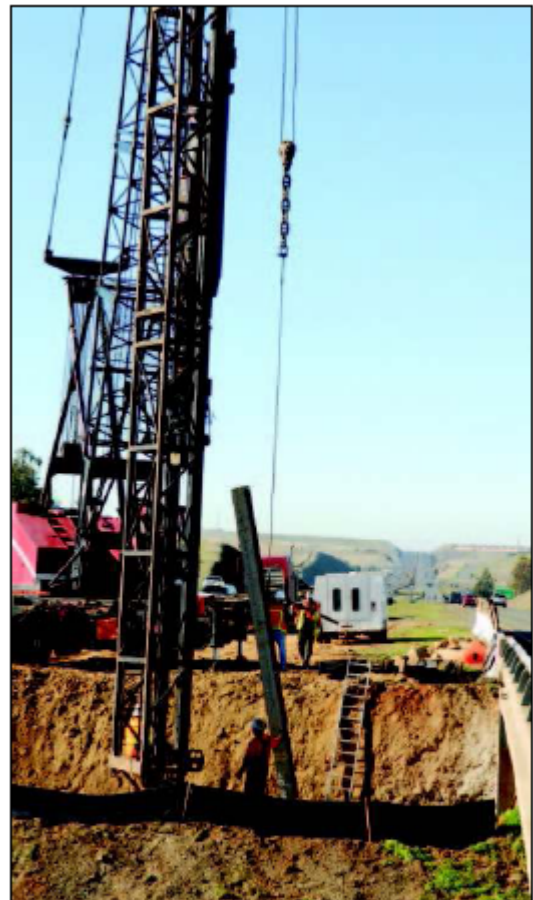
Mother Lode News photos by Pat Dollins HEAVY DUTY — Workers prepare a pile driver at the Highway 50 overcrossing of Silva Valley Parkway. The 1,500-pound piles are needed for the bridge expansion abutments that will accommodate carpool lanes on the freeway.
