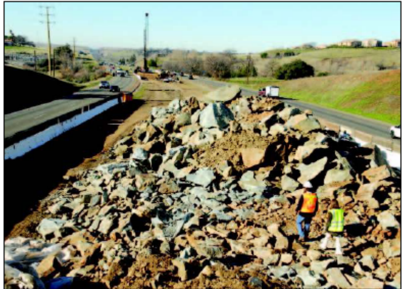
JOHN KAHLING OF DOT and a Village Life reporter pick their way through rock that has been broken up by Nehemiah Construction to make way for carpool lanes from El Dorado Hills Boulevard to Bass Lake Road.
