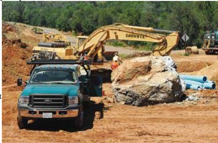
ORIGINALLY BOXCAR-SIZED when it taxed crews trying to unearth it at Shingle Springs Rancheria, a boulder now truck-sized after crews chopped on it is part of the construction site terrain where a Foothill Oaks Casino will stand. See story “Road ...”
