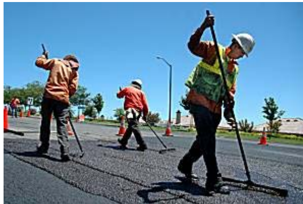
Javier Pahuia, from left, Asunzio Guitierrez and Sergio Guitierrez smooth out asphalt placed on Serrano Parkway, one of the EDH roads getting much needed attention. Robert Scott/The Telegraph
